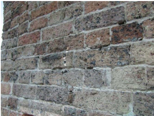
DETAIL OF THE SANDSTOCK BRICK WALL SHOWING DEGRADED SURFACE
