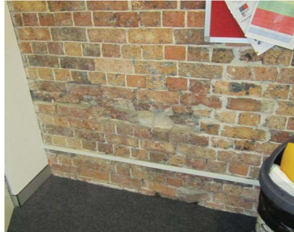
DETAIL OF FAILED AND DAMAGED BRICKWORK AT THE WESTERN END OF THE CENTRAL WALL (NORTH STORE)
