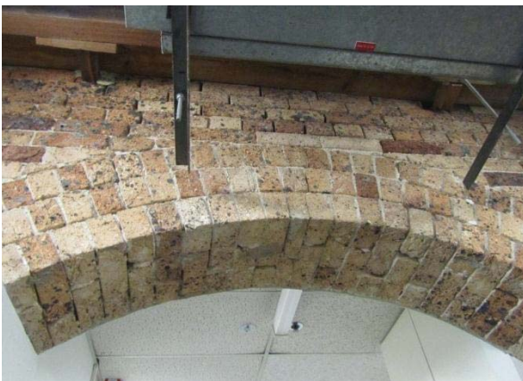
THE CENTRAL ARCH BETWEEN THE STORES HAS MISSING MORTAR AND JOINTS AND REQUIRES SOME ASSESSMENT
