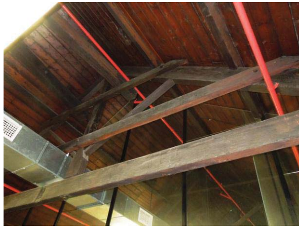
THE KING POST TRUSS ROOF, REINFORCED IN ASSOCIATION WITH THE EXTANT FAÇADE PULLEYS
