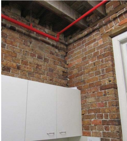
CRACKED BRICKWORK, MISSING MORTAR AND OPEN JOINT INDICATES MOVEMENT IN THE WESTERN ELEVATION AT THE JUNCTURE OF THE CENTRAL WALL (NORTH STORE)
