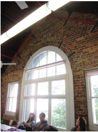
THE EASTERN ELEVATION GABLE SHOWING STEEL REINFORCEMENT OF ARCHED BRICKWORK AND ROOF.
