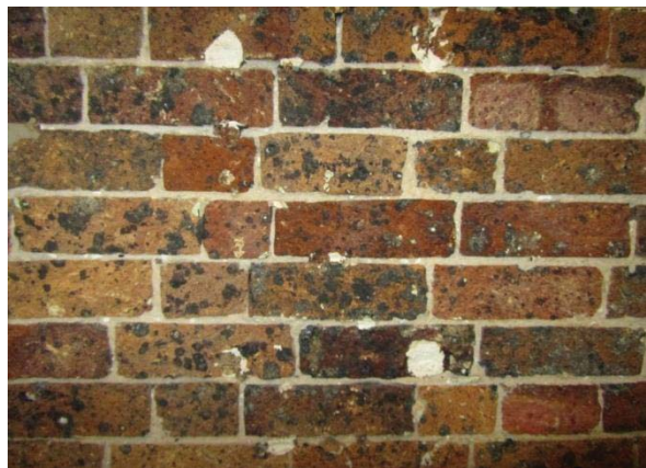
DETAIL OF THE SANDSTOCK BRICK WHICH HAS BEEN DAMAGED IN CONJUNCTION WITH THE REMOVAL OF RENDER AND FINISHES
