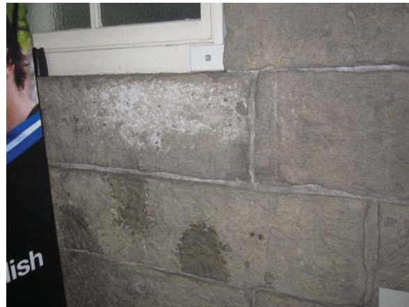
DETAIL OF THE NORTHERN WALL SANDSTONE SHOWING EVIDENCE OF SALT ACTIVITY AND CEMENT PATCHING
