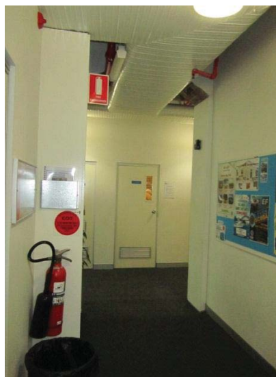
VIEW NORTH, ADJACENT TO THE STAIR HALL AND SHOWING CONTEMPORARY DUCTING AND SERVICES
