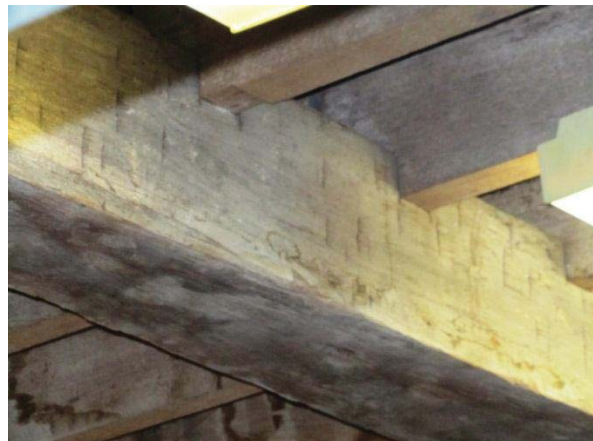
DETAIL OF ONE OF THE SUPPORT BEAMS WITH FLOOR JOISTS OVER. THE BEAM IS HAND ADZED WITH TOOL MARKS EVIDENT (SOUTHERN STORE).
